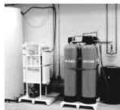
Pro Ice Reverse Osmosis Water Treatment
