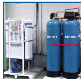
Pro Ice Reverse Osmosis Water Treatment
