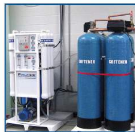
Pro Ice Reverse Osmosis Water Treatment
