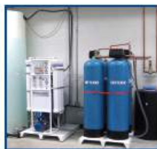
Pro-Ice Reverse Osmosis Water Treatment
