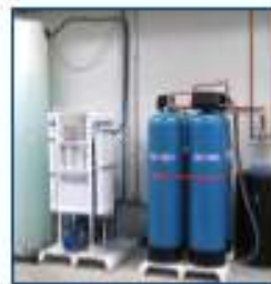
Pro-Ice Reverse Osmosis Water Treatment
